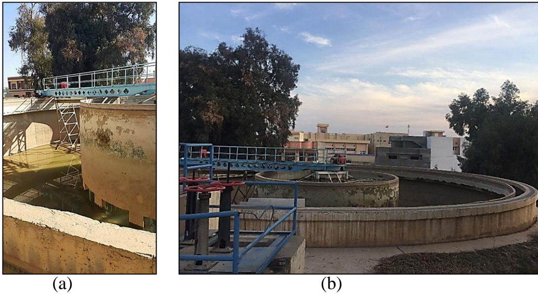
Figure 3, (a and b). Flocculation – Sedimentation basin at KCWTP
